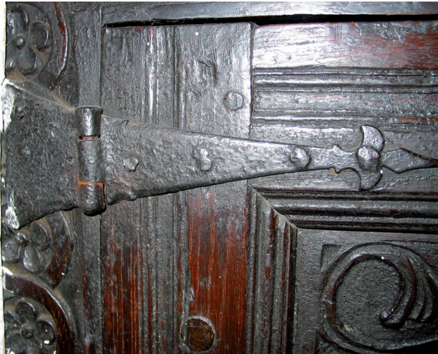
15 Hinge detail, showing surface mounted metal hinge, Bannerigg Farm. The National Trust
